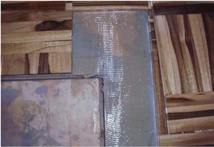
Top picture; combed adhesive, middle and bottom; first coat of sealer going down
